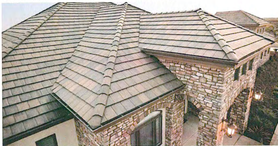
Photo Y: Narrow fascias at the roof overhang
